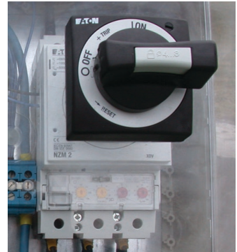
Kemper has installed Eaton's NZMN2-VE250 circuit breaker in a prominent position on the dashboard. In this image, it is combined with a turning handle to switch it on and off (source: Kemper)
